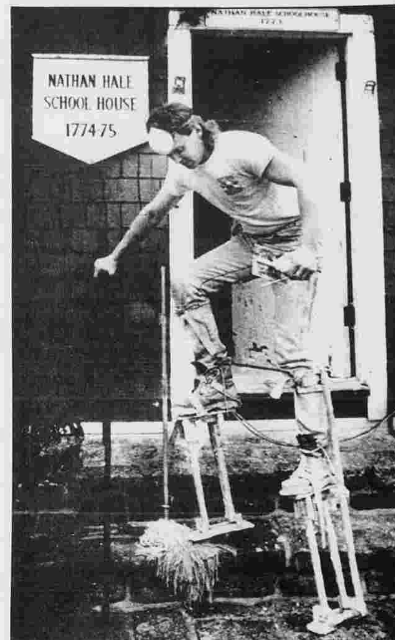
HIGH-STEPPER — Plasterer Scott Awker steps cautiously out of a work site in New London Tuesday for a breath of fresh air. Awker uses the stilts because, he says, they are more convenient than working on a step ladder.
